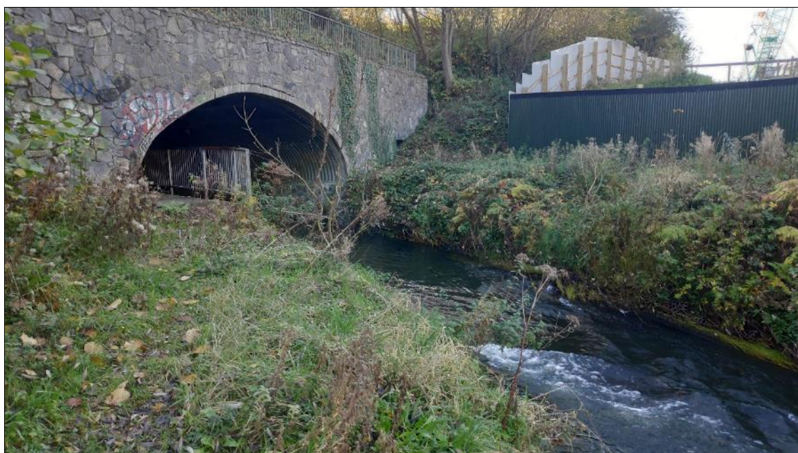
Plate 3.2 Representative image of site T2 on the River Tolka (facing upstream towards culvert)
